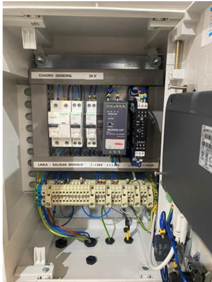
Figure 14: Image of the electrical panel.
