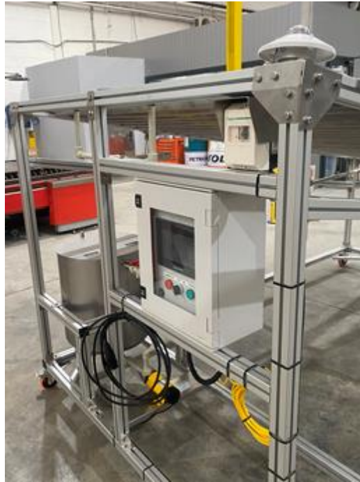
Figure 17: Image of the different electric components
