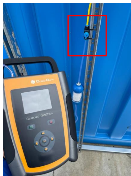
Figure 2. Biogas analyser connected to sampling point when manual valve is open
