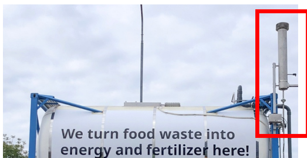
Figure 6. Flare System (top right)
