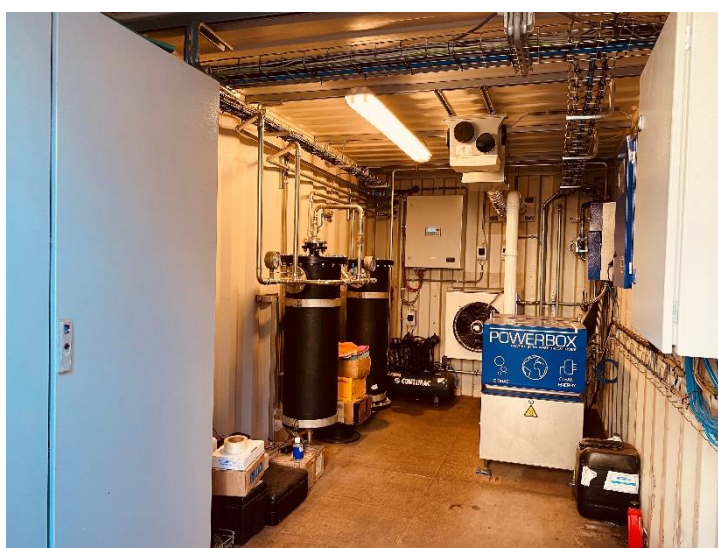
Photo of the electricity generation compartment of the biodigester system being installed in Freetown Sierra Leone
